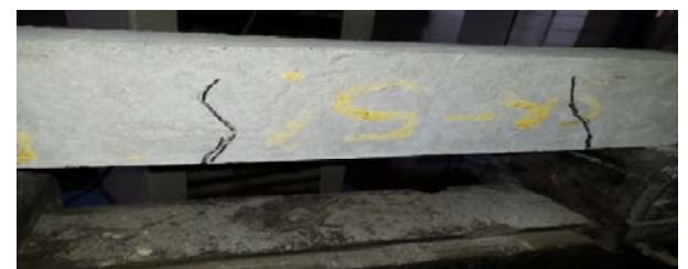
Figure 30 Beam failure combinations of (flexure and shear)
